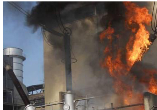
(b) Bushing Explosion [17]
