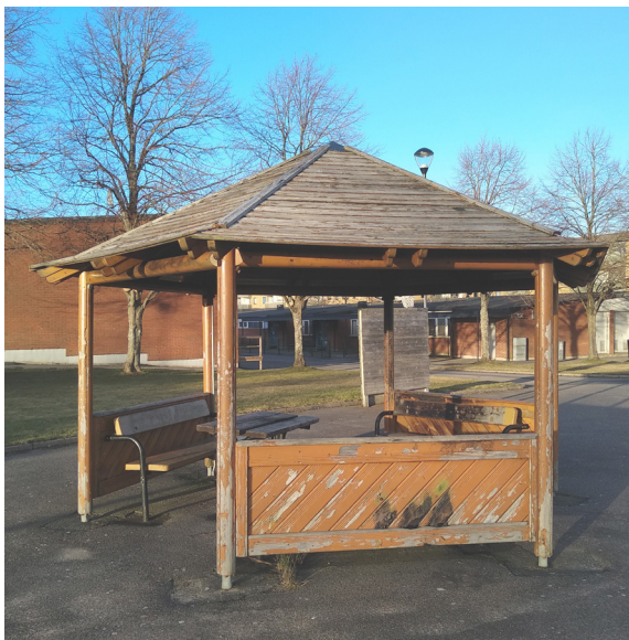
The old gazebo in a bad condition.
