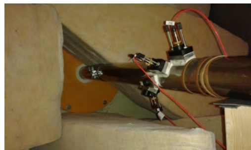
(h) Mounted in-duct microphones at the inlet.
