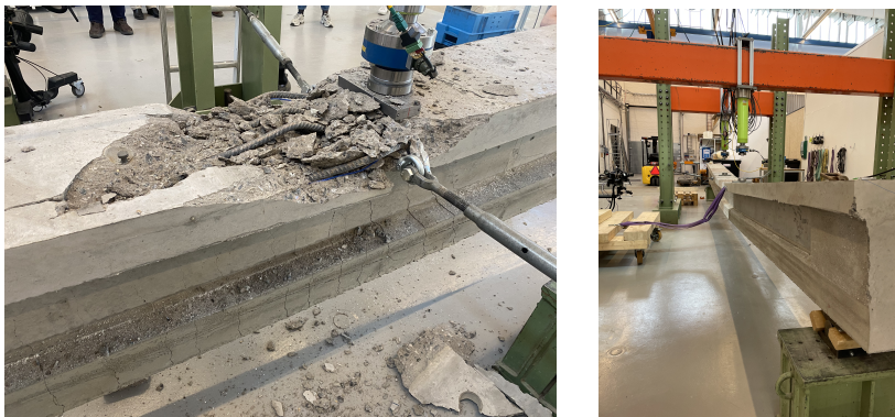
(a) Failure of PRC specimen.
