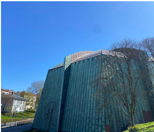
Figure 2. The building “Kopparbunken” at Johanneberg as an example of copper roofing showing signs of corrosion.
