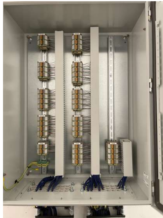
(b) View of cable management inside cabinet.
