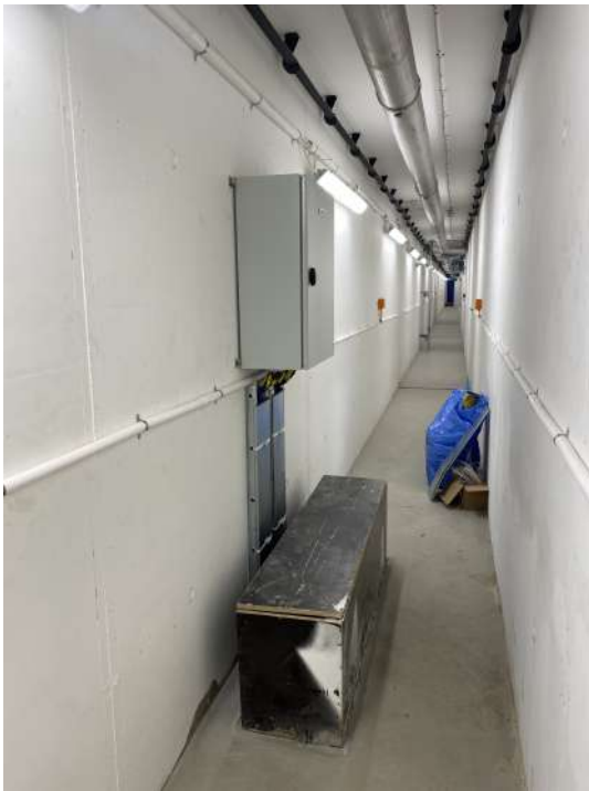
(a) Location of electrical cabinet.
