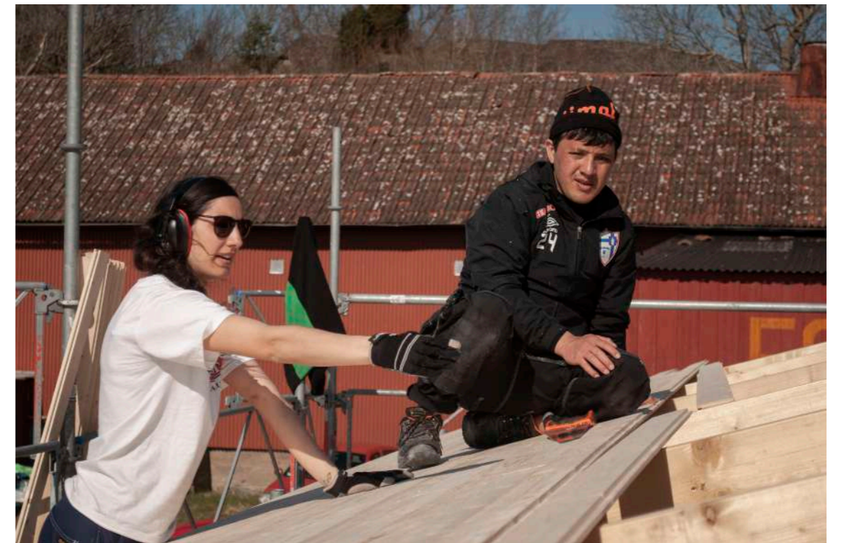
Image 54. Construction of the roof took several sunny days with appreciated help from a carpenter and a volunteer. April 6
