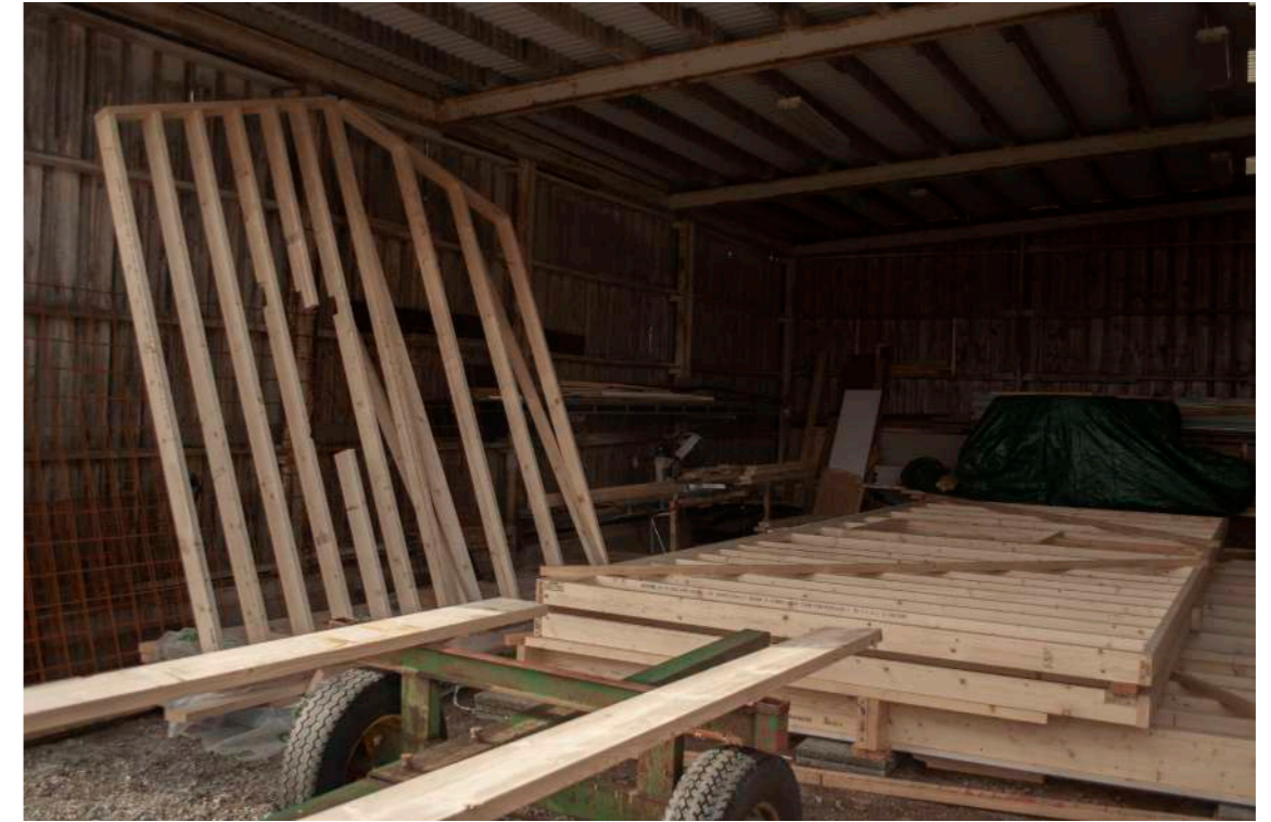
Image 34. Moving out the structure. The client was visiting the construction when moving which made the moving of the structure easier. March 24
