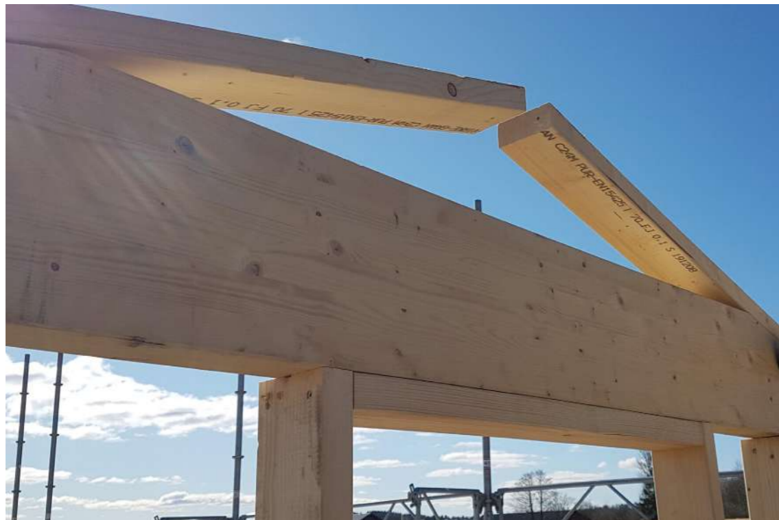
Image 45. Mounting of the unloading beam which was sawn from the ridge beam. March 30
