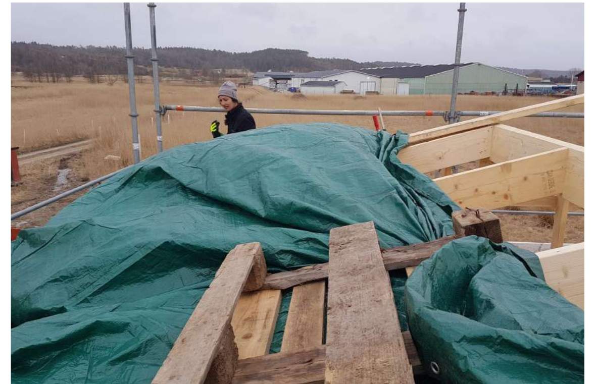
Image 53. The tongue and groove is very sensitive to wetness. A storm warning had been announced and it took 1.5 hours to secure a tarpaulin. April 1
