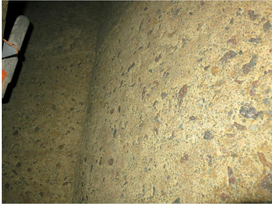
Figure 3: Damage due to leaching (photo: Anders Lindvall).
