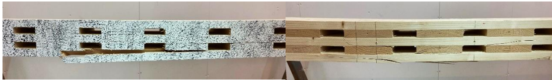
Figure 4-49 Detailed pictures of the failure for Sample 3 of Configuration B. The picture at the left depicts the front side and the right one shows the unpainted backside of the beam.
