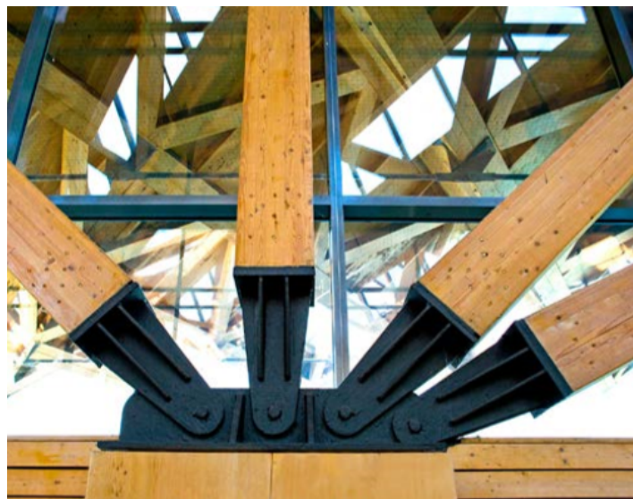
Figure 2.7: A complex timber-steel connection to obtain a hinged boundary condition. Photo © Åke E:son Lindman
