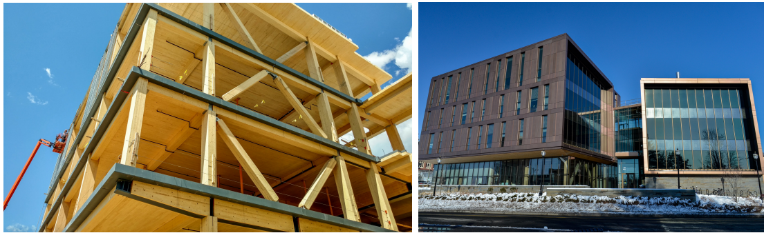
Figure 4.11: Left: picture of the timber structure. Right: picture of the finished building. Photos © Alex Schreyer / UMass
