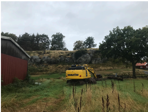
(c) Photo of excavator showing the building, tree and the terrain near it.
