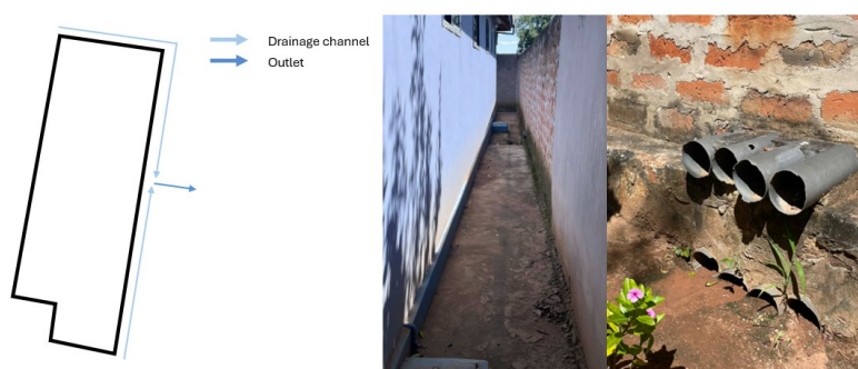
Figure 5.7: Left: Layout of the volunteers' house indicating the location of the drainage channel and outlet. Middle: Open drainage channel along the backside of the building conveying greywater. Right: Outlet pipes discharging greywater from the channel to the surrounding planting areas outside Area III.
