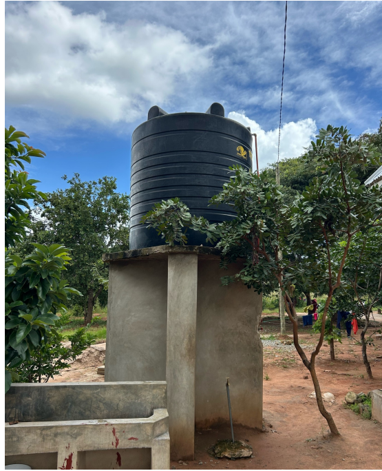
Figure 5.23: Existing municipal water storage tank at Tumaini Open School (5 m 3 ).
