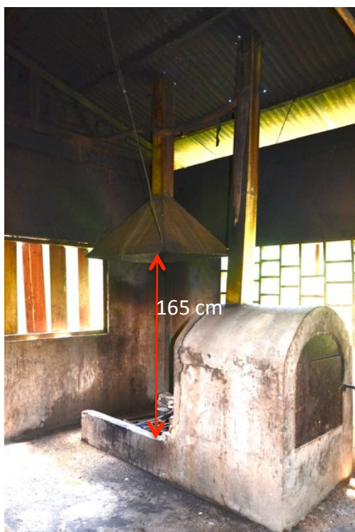
Figure 7: Installed chimney in another village called Puerto Triunfo
