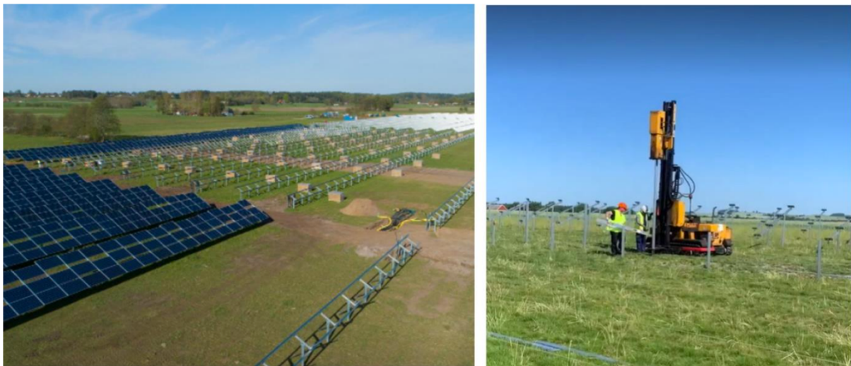
Figure 2.3 Imagery illustrating installation of a typical GMPV in Sjöbo, southern Sweden (OX2, 2023).
