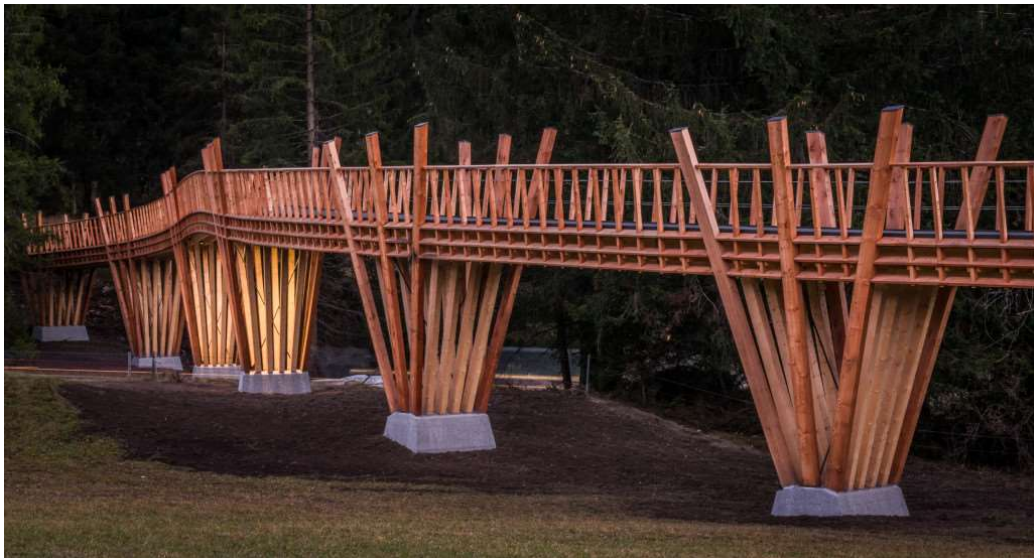
Figure 3.6 Side view of Punt Staderas (Camathias SA, 2015a). Note the cover board that leads water away from the structure. Used with permission.
