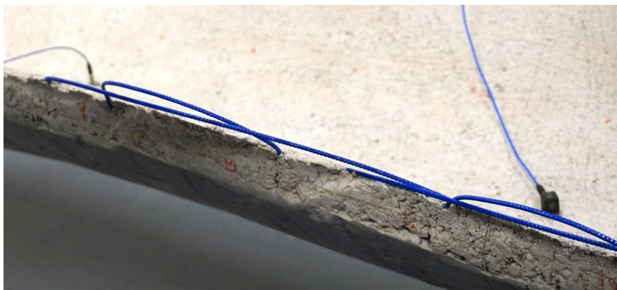
Figure 3.9: Honeycombing along edges.
