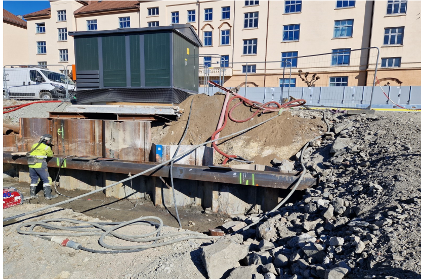
Figure 4.4. The cable from the excavator lying on the ground and connected to the substation. Own photograph.
