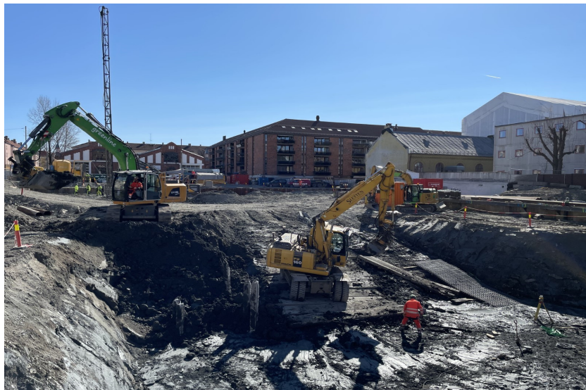
Figure 4.5. The electric cable excavator, the HVO excavator, and a construction worker operating hand-held machinery. Own photograph.
