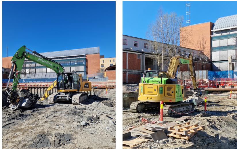
Figure 4.2. The two electrical machinery used in the project. 26-ton cable crawler excavator (Left), 10-ton battery crawler excavator (Right). Own photographs.
