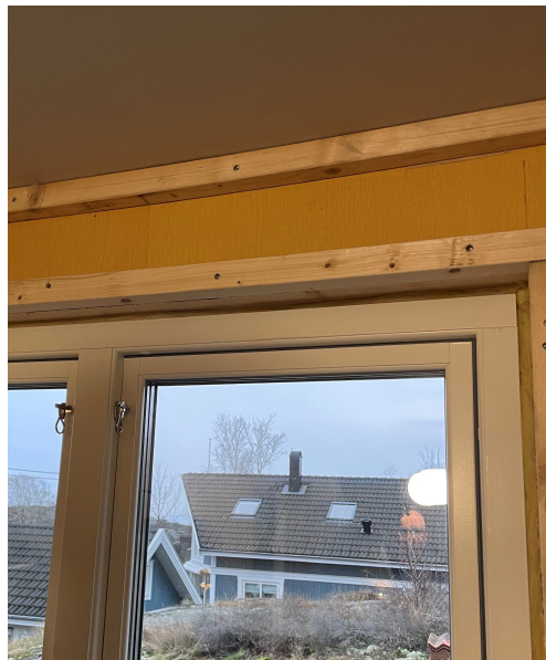
Figure 4.13: Example of how it can look as first sight for an electrician
