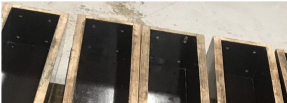
Figure 7.2 Sample of moulds showing bored holes to give space and support for rebars.
