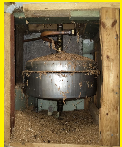
Expansions tank for water circulation in the radiators.
