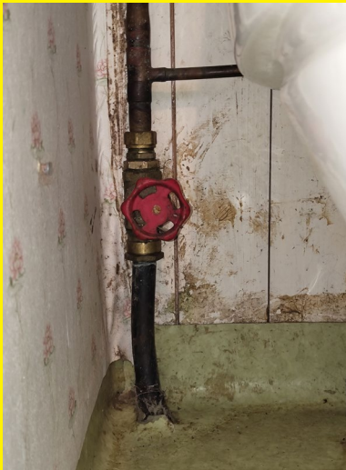
The water intake pipe in the bathroom.
