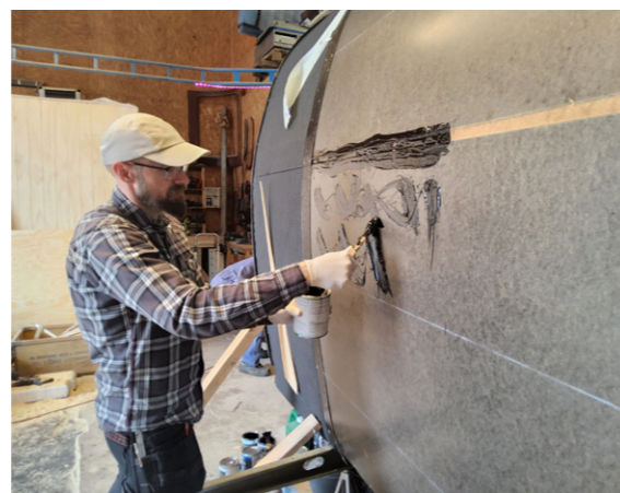
Figure 49: We struggle to attach the roofing felt on the sides, but do our best with asphalt glue.
