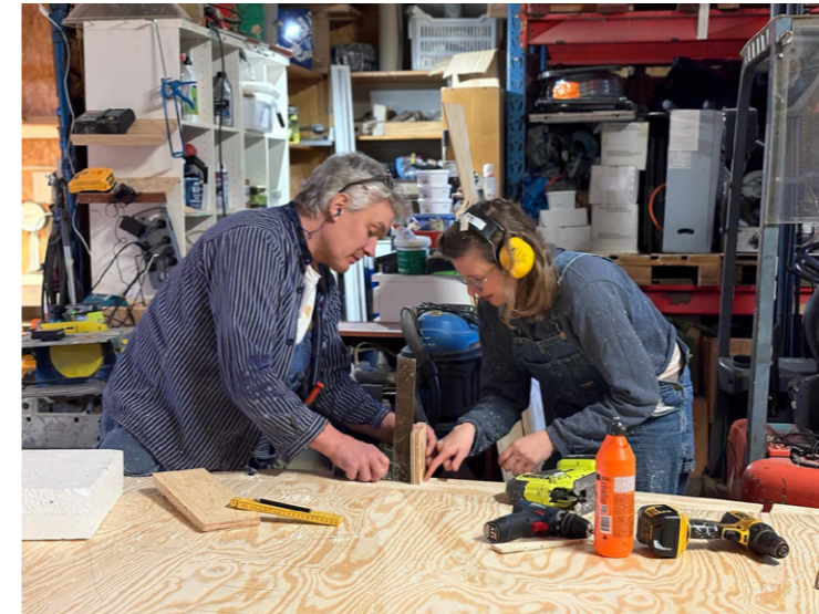
Figure 46: Us teachers had to help out to make it in time. Work was progressing slowly with the self-builders, which leads me to see the role of professionals in a more positive light.
