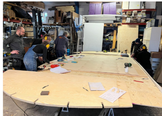
Figure 43: We cut the 4 sheets of plywood used on the exterior and interior walls at the same time.
