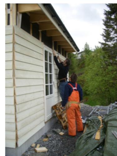
Figure 14: In the government-initiated project in Meland, Norway in 2008, youth with a history of criminality or addiction were invited to build their own house (Lundquist, 2017). The municipality allocated cheap land and unemployed carpenter students provided tutorials. The hope was for the participants to be provided with a way to change their way of life for the better. Attempts were made to calculate the social benefit of the project. Based on the fact that a person in active criminality costs society about 19 000 NOK per day, and 5 such people completely stopped their criminal activity for the 5 years the research covered, means a societal saving of 200 million NOK (Hansen et al., 2009). The gains for the participants in terms of a place to live, increased sense of self-worth and useful skills are of course immeasurable.
