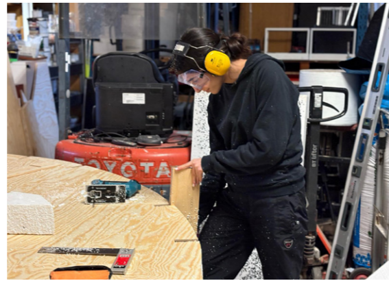
Figure 60: We had to spend a lot of time correcting mistakes, such as cutting bigger jigs in the facade for the roof rafters to fit.
