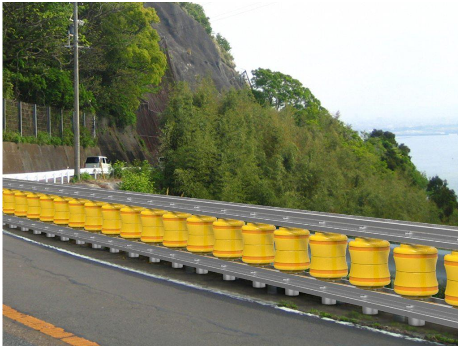
Figur 38. Rolling Barrier Guardrail.
