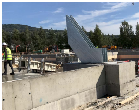
Figure 1.3: Image of the massive slotted-in steel plates of timber connections used within the Mjøsa Tower. Source: Images from the presentation by CEO of Moelven Limtre, Rune Abrahamsen, at the Internationales Holzbau-Forum IHF in 2017
