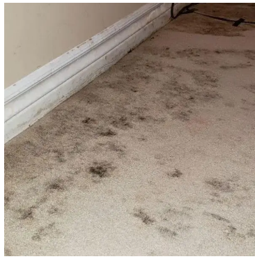
(a) Mold, mildew or rot buildup on carpets and wooden structures [71].
