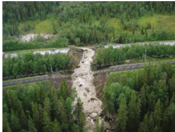
Figure 2: In summer 2006, a road and rail embankment was washed away at Änn in Jämtland after intensive rain upstream, resulting in a high flow and erosion.
