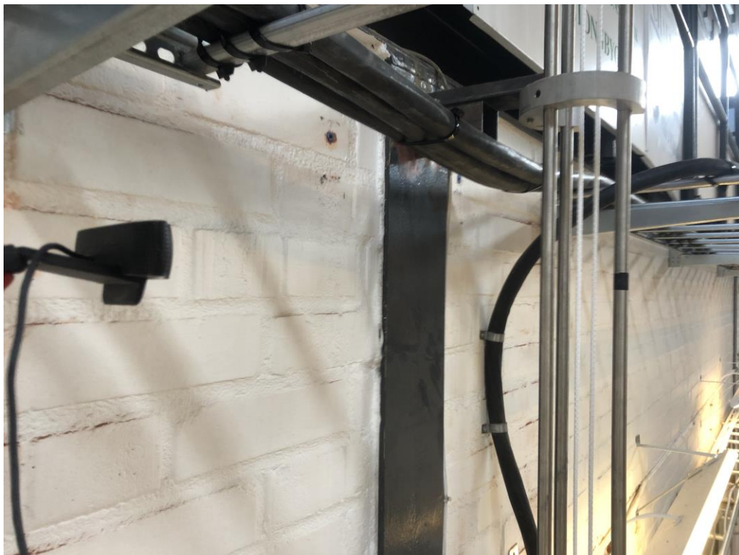
Figure 8.24 Web camera set-up showing camera placement and height marking on the guiding tube.
