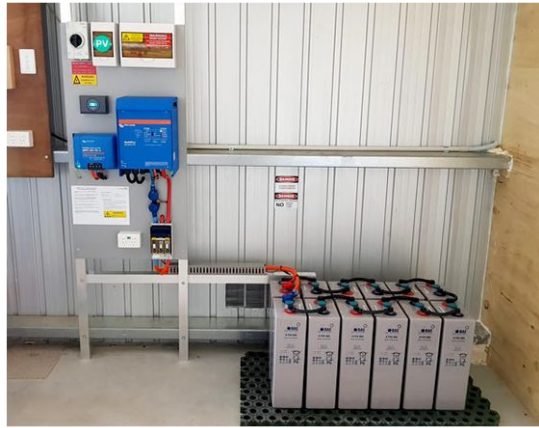
Figure 1.1: Residential solar-battery system with wall-mounted inverter and battery bank.[1]
