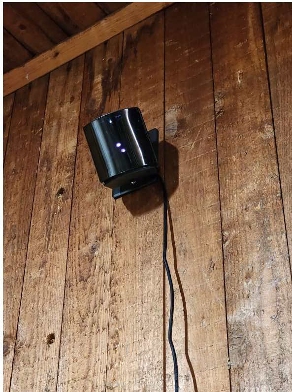
Figure 3.9: Installed base station
