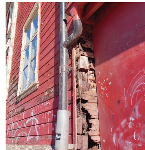
Heavy disrepair, Bangatan March 2022
