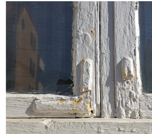
Careless renovation, Bangatan March 2022
