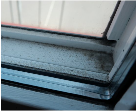
Figure 49: Interior window condition in school 1
