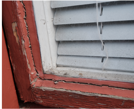
Figure 50: Exterior window condition in school 1
