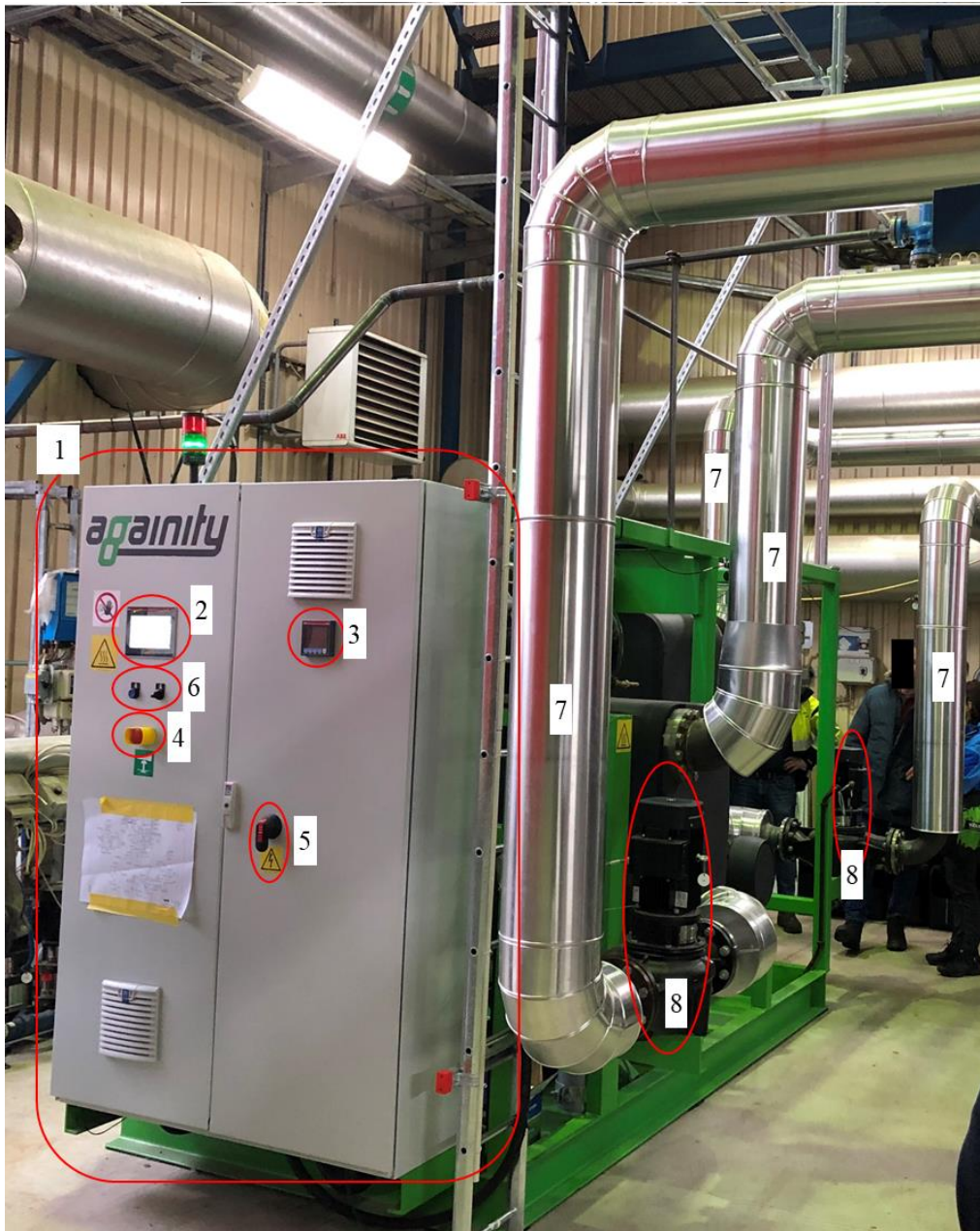
Figure 43: Smallest ORC unit from Againty AB capable of producing 50 kW el installed at Alvesta Energi (Picture personally taken by author and copyright given by personal correspondence with Againty).
