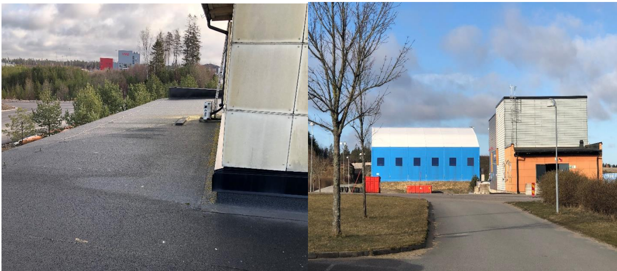
Figure 10: Lower roof level of weighing station building (left) and water treatment building and temporary storage of unknown soils tent at the back (right).
