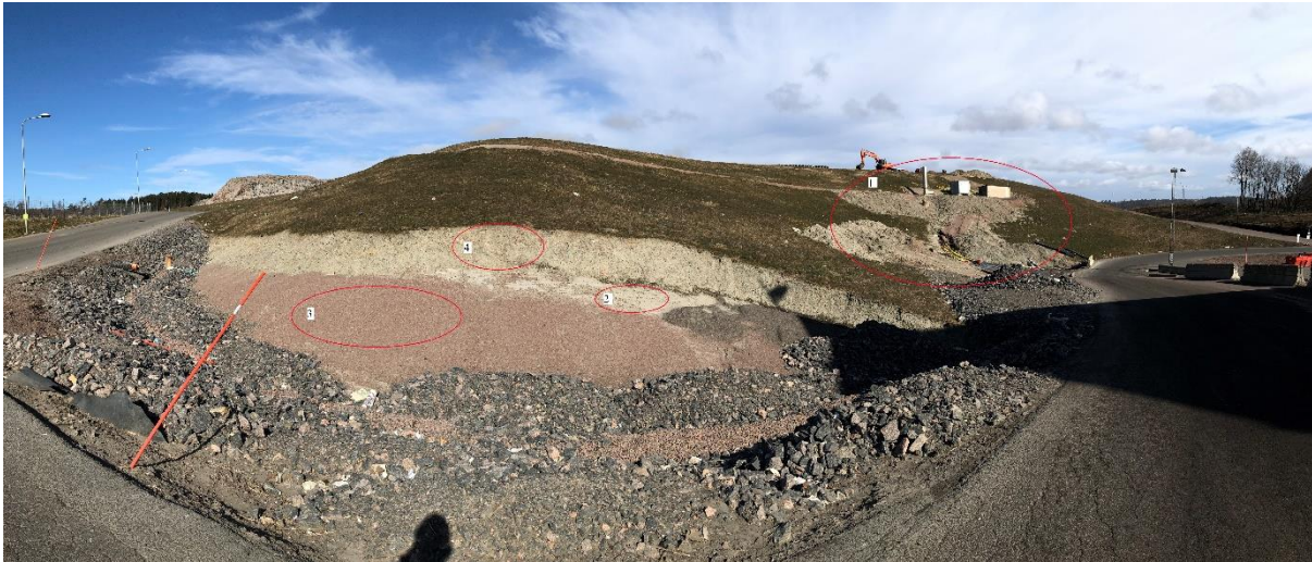
Figure 19: Panoramic image showing the moved flaring station and the road work done at the bend of the road.
