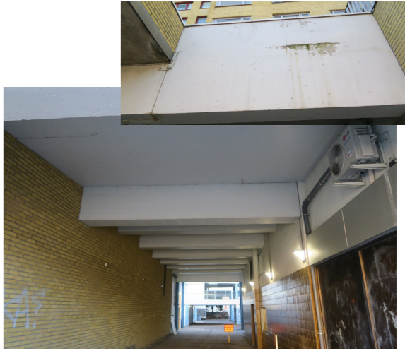
Ceiling consists of a beam rhythm. Some parts feels dirty and damaged.
