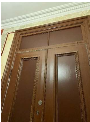
Figure 22 The door is neither modern nor original.
