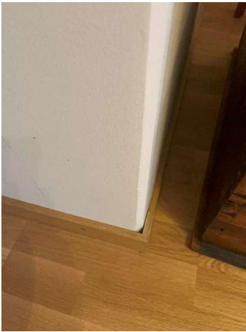
Figure 27 The residents found a lack of care taken to details in construction. Gaps between skirting boards and wall being one of them.
