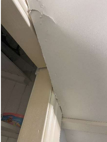
Figure 36 If something looks strange or is poorly constructed, it is not the original construction.
