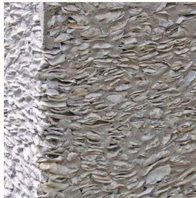
Tabby concrete with whole oyster shells as aggregate. Image source: Rory Gardiner
