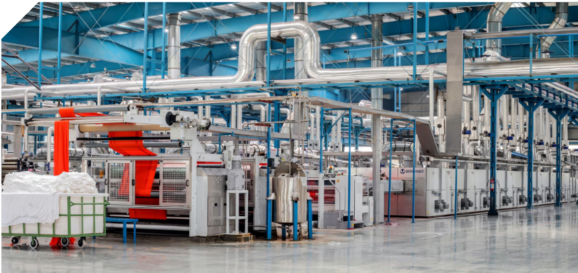
Figure 4.2. Example picture of what the layout of a company within the engine industry could look like.
