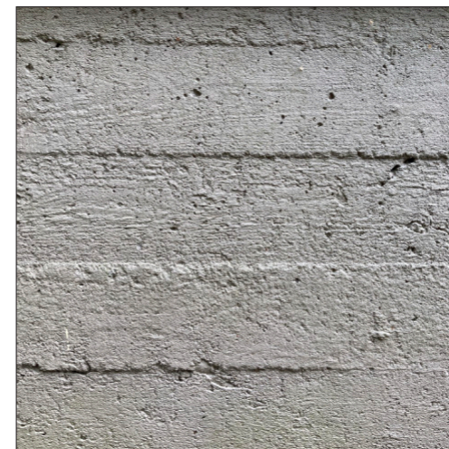
Timber formwork was use as mould for the reinforced concrete foundation. The boards used are still saved as flooring in the attic, as seen in figure ?.
