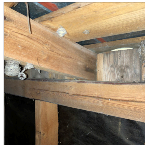
Boards to support the sheet metal roofing were placed sparingly with varying distance.
