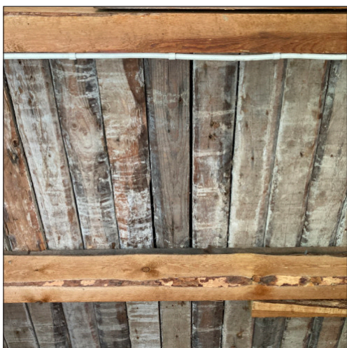
Everything was used. The timber from the formwork was used as flooring on the attic. Traces of concrete are clearly visible. These could be reused in future formwork.
