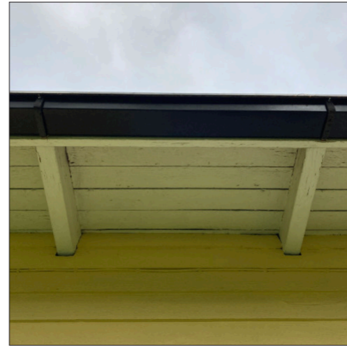
The building has been fitted with a square type water drainage and the distance between the roof beams is around 920 mm.
