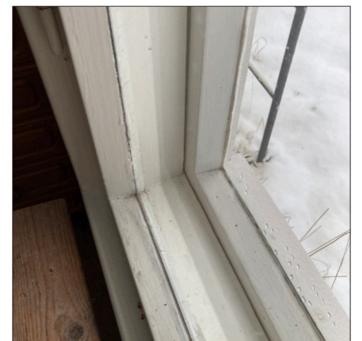
Window arches are almost as deep as the external wall and are made up of two single sashes.
