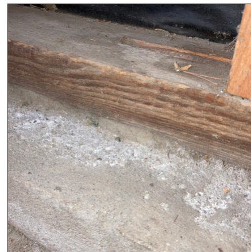
There is no vapor barrier between the concrete foundation and the timber sole plate. Only a strip of mineral wool was used to separate the timber structure from the foundation.
