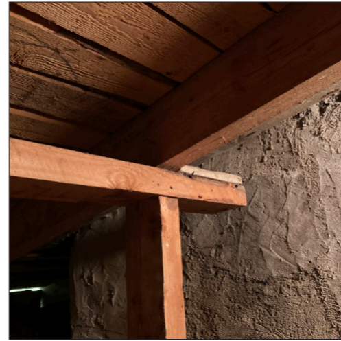
Simple support of the roof beams, sawn where necessary to make room for the chimneys.
