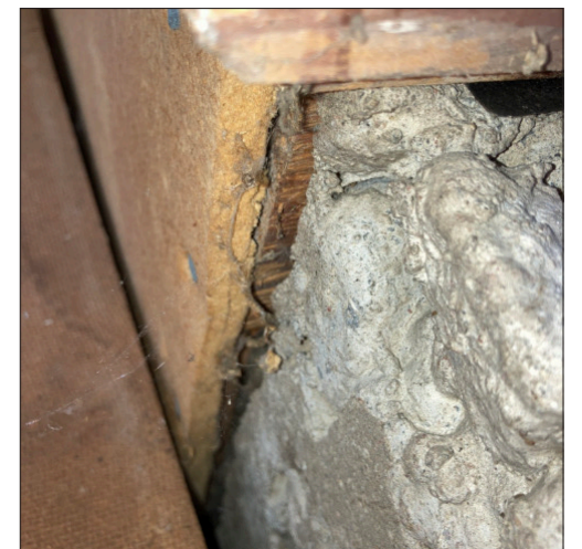
At some points there seems to be nothing separating the timber sole plate from the foundation.
