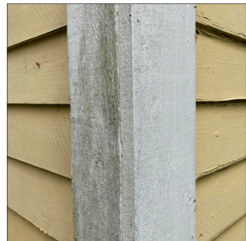
The corners are covered with timber, organic growth is evident on most parts of the building that has been painted in white.
