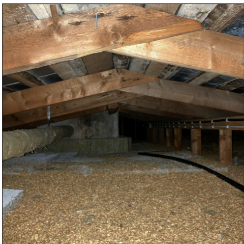
Sawdust was used as primary insulation. Over time some fireproofing insulation and cellulose insulation has been added. The sawdust layer is about 300 mm thick and the roof beams have a 65x130 mm dimension.
