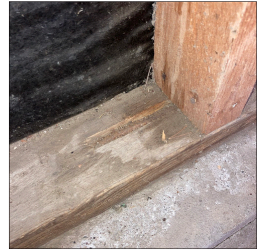
The timber sole plate is anchored to the concrete foundation with a bent 10 mm rebar.
