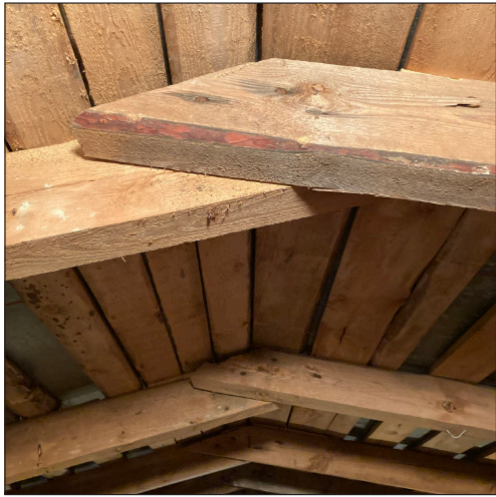
Roof beams were placed side by side and nailed together. No ridge beam was used. To support the roof two beams with studs running parallel on both sides along the ridge were used. Roof angle is about 12 degrees.
