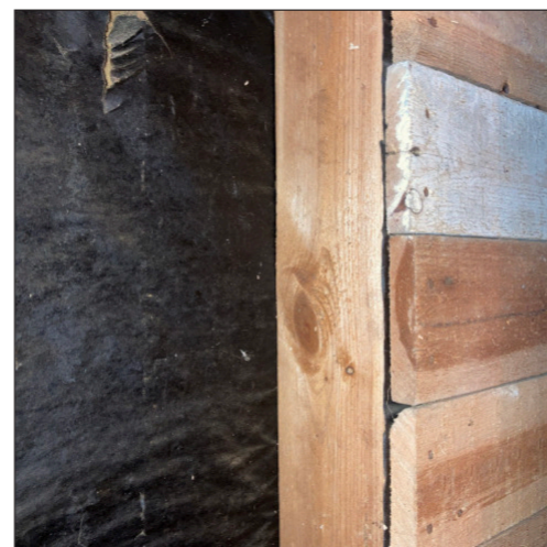
Exterior wall is made up of 100x50 mm studs, clad with bituminous paper and timber boards. Space between studs was filled with sawdust insulation which later was replaced with mineral wool, particularly under windows.
