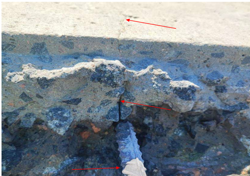
Figure 3.17: Close up of the crack extending to the bar surface from Afry reports.
