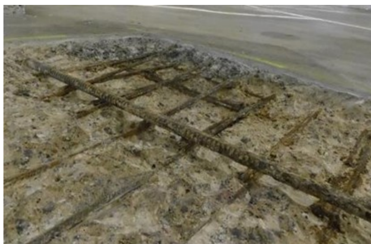
Figure 3.10: Status of the bars in the window F2 from Afry reports.
