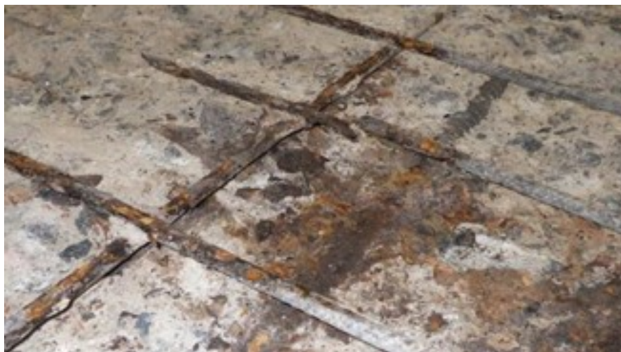
Figure 3.7: Condition of the reinforcement in the Window F1 from Afry reports.
