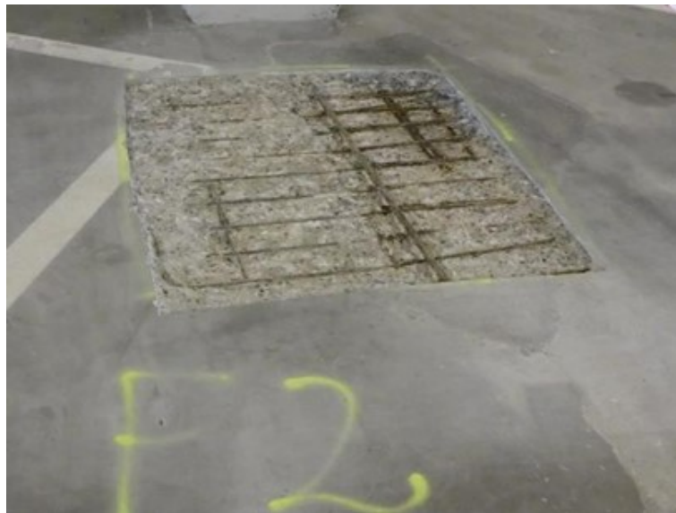
Figure 3.9: Status of the bars in the window F2 from Afry reports.
