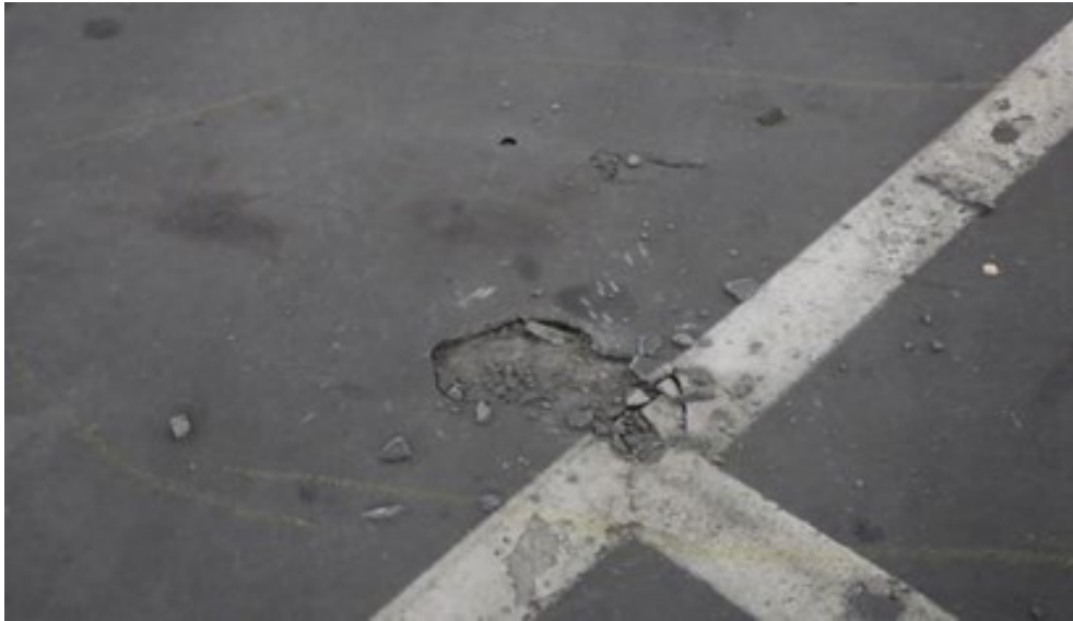
Figure 3.2: Cracks and concrete spalling in the upper section from Afry reports.
