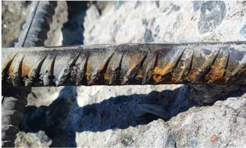
Figure 3.16: Localised corrosion close to the cracks in window F2 from Afry reports.
