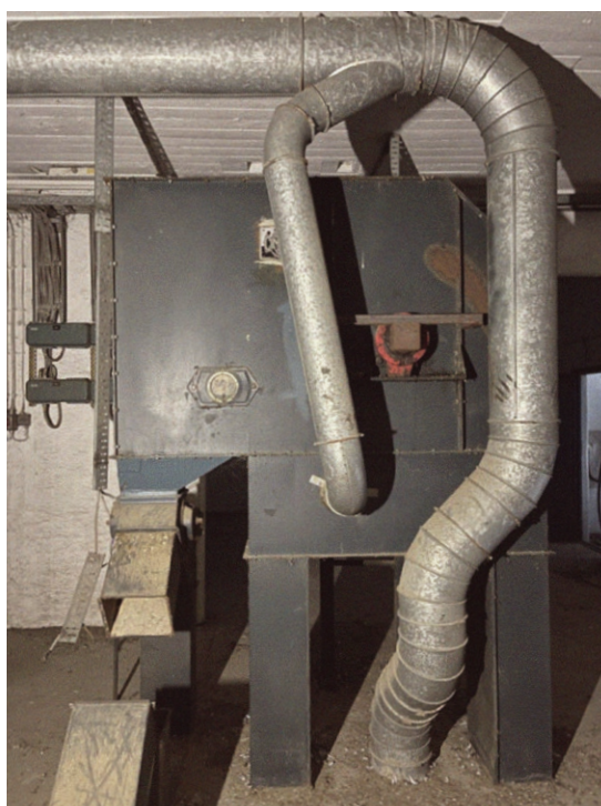
Figure 40. Interior photograph, machinery.
