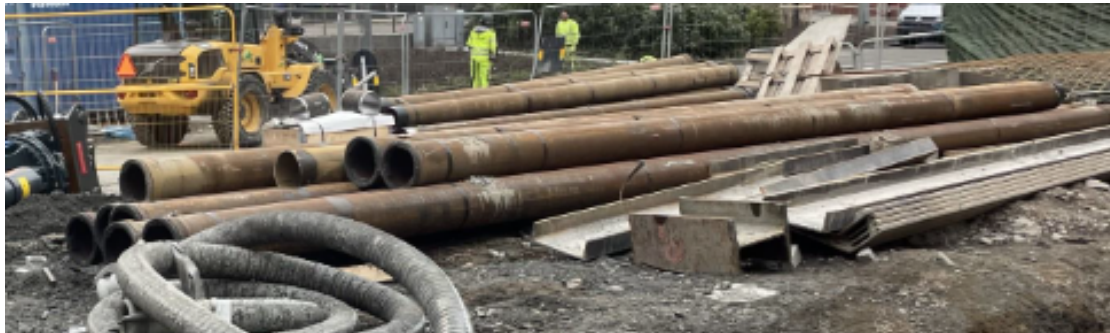
Figure 2.7: Picture taken on-site of drilled piles used at the Sahlgrenska life project. Own image.
