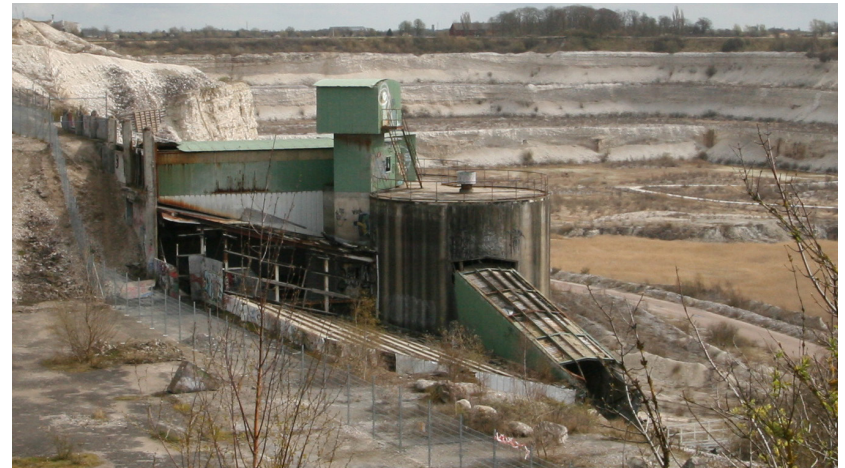
Figure 25. The silo roof is at sea level +0 and reaches up above the plateau at -6m. Remnants of conveyor belts and structures covering the gap in-between the silos and the limestone wall are in poor condition.
