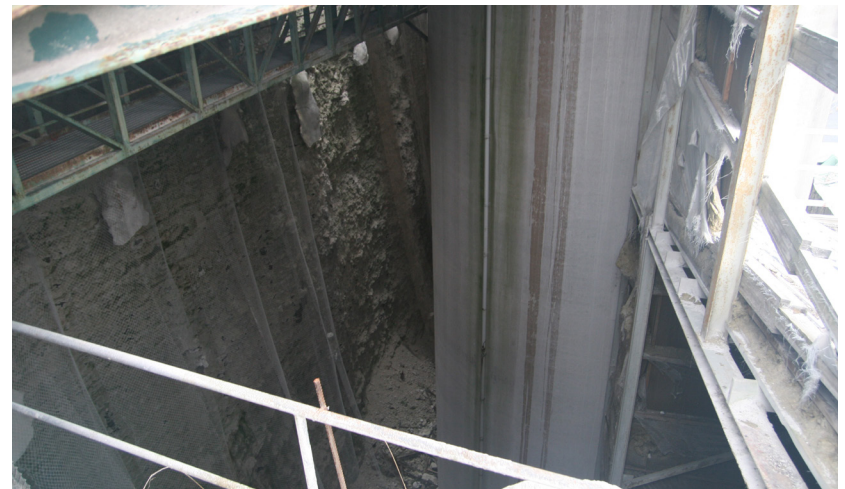
Figure 26. View of the space in-between the silos and the limestone wall. The silos appear to be in good condition. The structures around the silos are falling apart.
