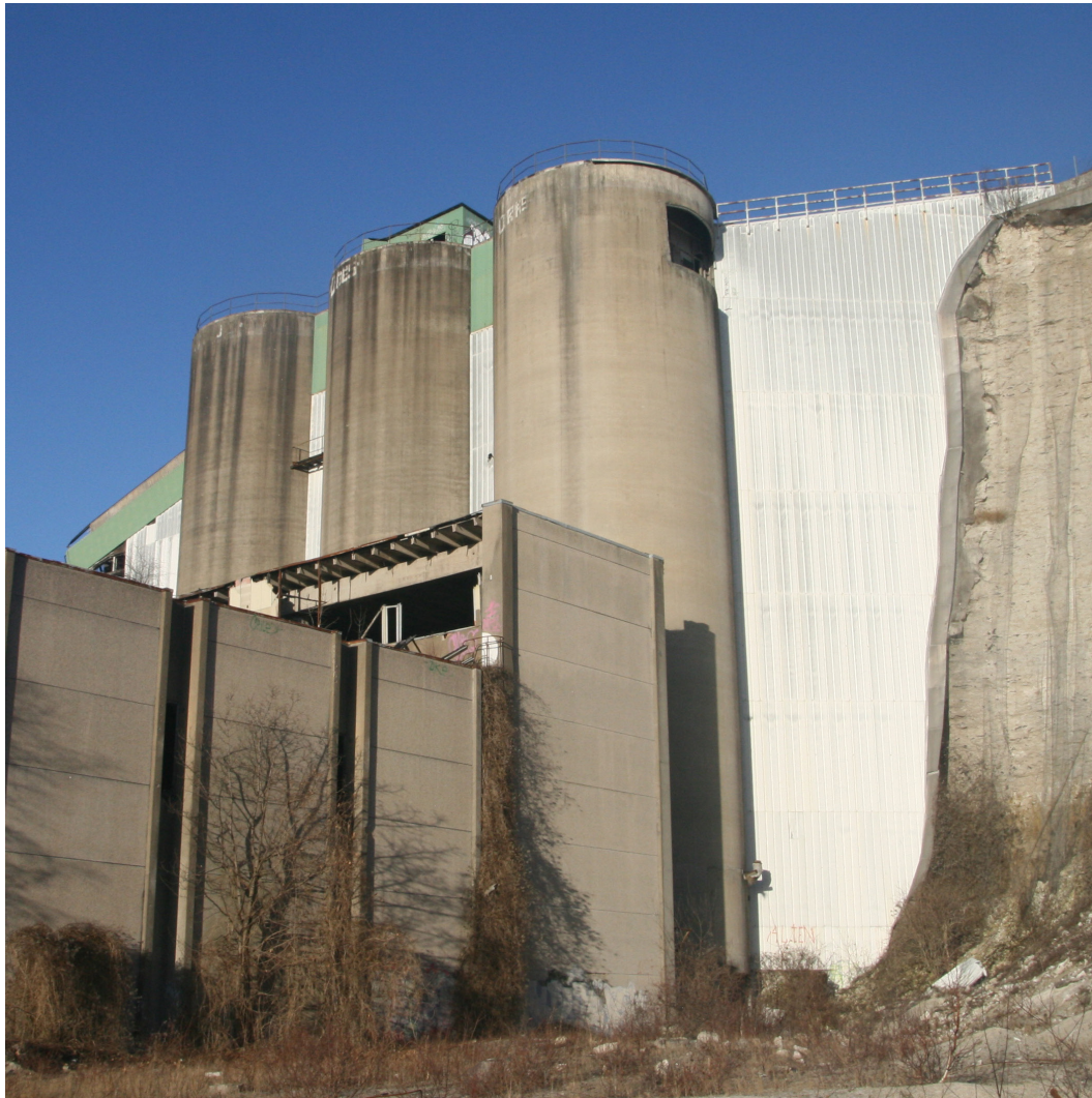
Figure 24. The building in front of the silos was used for crushing limestone, it has a partly demolished operator room on the roof. The load-bearing structure of the stone crusher building has major frost damages. The gap between the silos and the limestone wall is covered with metal sheets.
