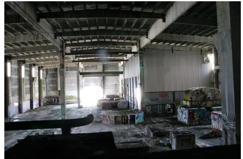
Figure 30. View from the balcony in front of the silos, the floor in the former stone crusher building is covered with large concrete bases.
