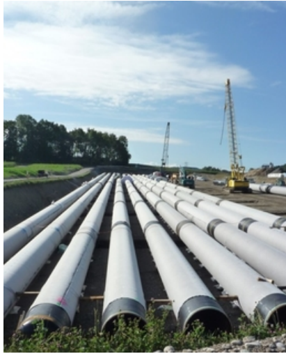
Figure 2: A photography of the 6112 m 3 natural gas pipe storage in Urdorf, Switzerland under construction [34].
