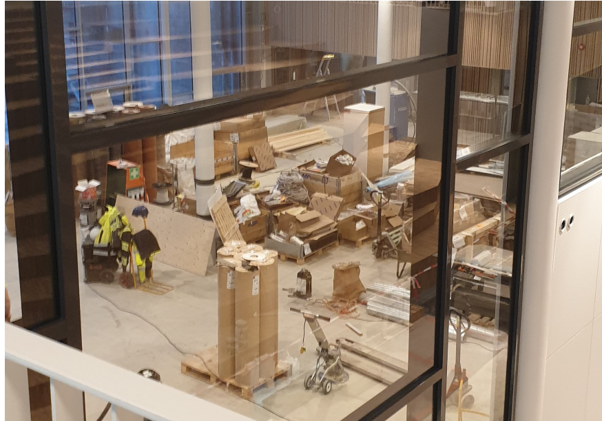
Figure 12: Photograph taken during a site visit, showing the future school canteen being used as temporary storage for goods requiring shelter from the weather.
