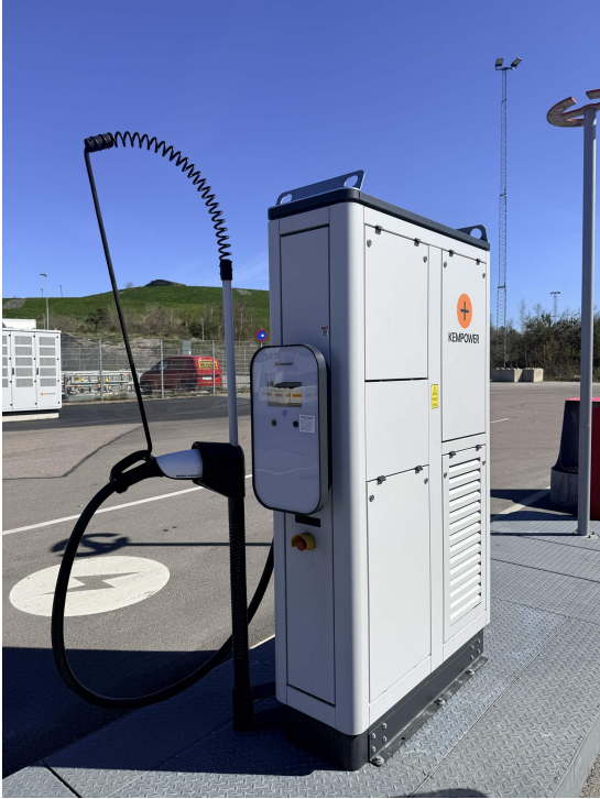
(a) MCS charging post.
