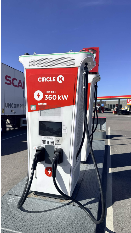
(a) CCS2 charging post.
