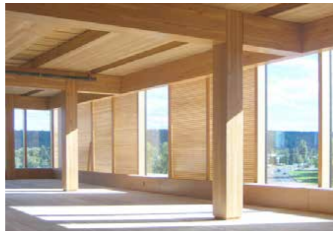
Figure 28. A way to allow exposed wood is to make posts and beams overly dimensioned and install a sprinkler system. (Archtonic, n.d.)
