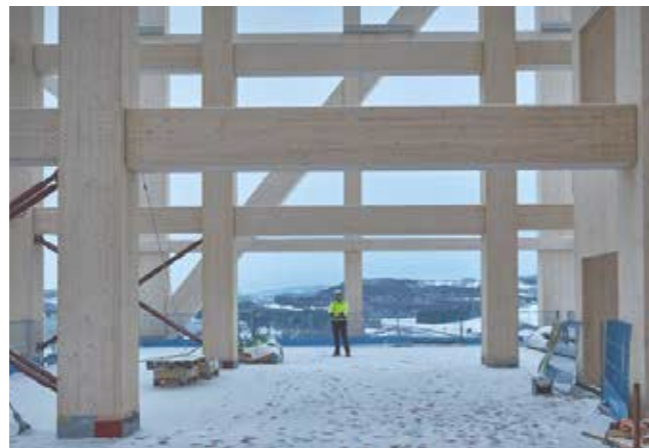
Figure 29. The structural system of Mjöstornet, the tallest wood structure in the world, is composed of glulam Posts and Beams, with lateral stability from glulam trusses (ArchDaily, 2018)
