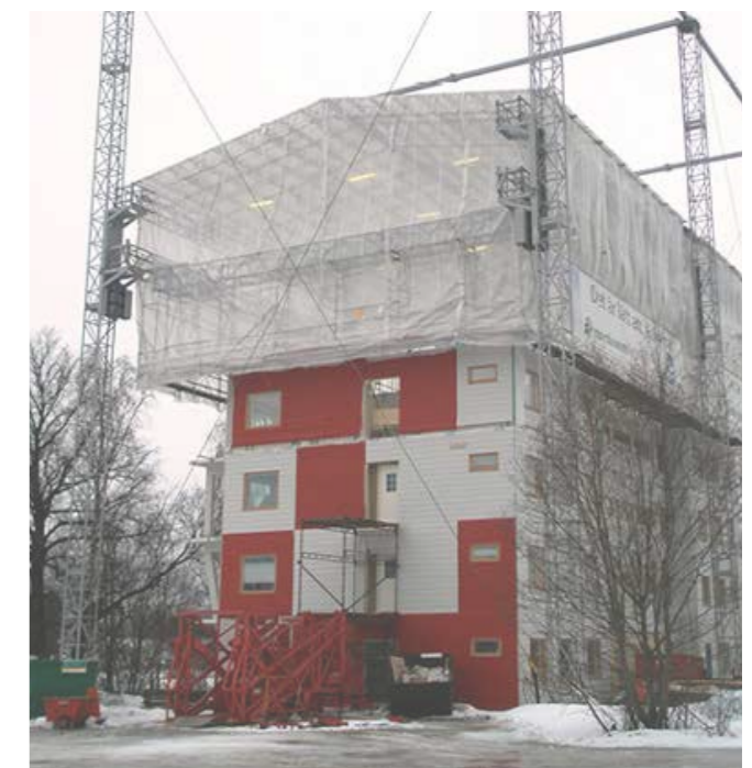
Figure 7. A weather protection on the building site can ensure a moisture free construction and give a shorter construction time. (Svenskt Trä, 2017)
