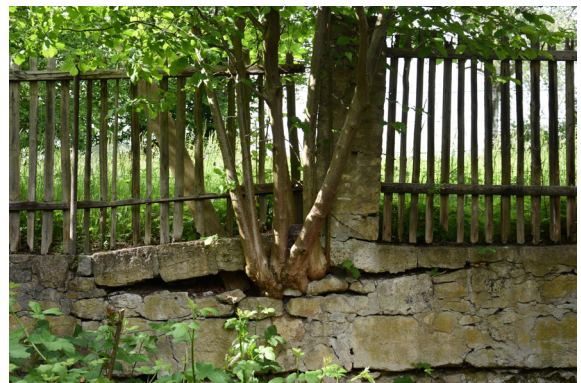
Figure 13 A hazel growing through a stone wall May 2022
