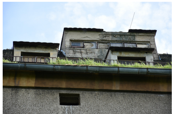
Figure 12 Grass growing on the roof of the silo May 2022
