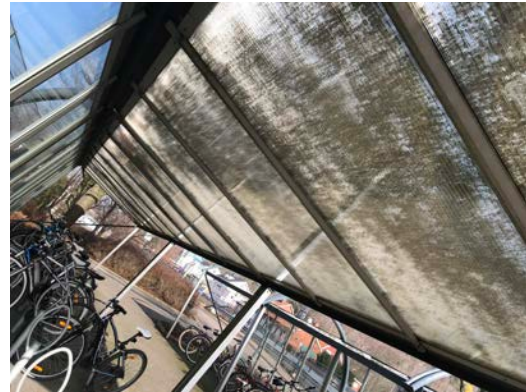
Figure 57. Dirty roof on bicycle shelter
