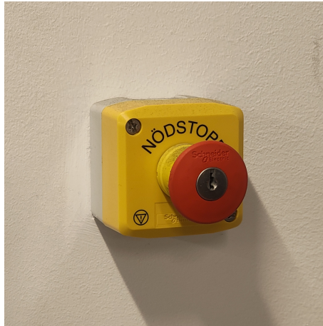
Figure 6.4: Example of an emergency stop button.
