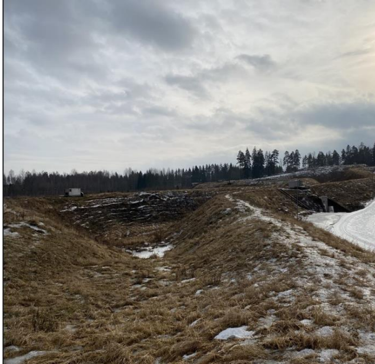
Figure 16: Figure showing Torsby ski tunnel from outside. Ground soil covering concrete structure.
