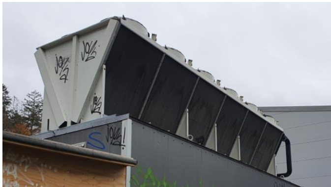
Figure 8: Dry coolers for the condensing process in the cooling machine.
