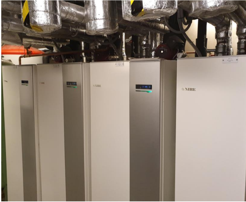
Figure 9: Heat pumps for comfort heating in Serneke arena.
