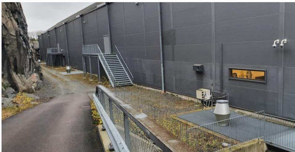
Figure 11: Three AHU located down in a ground pit outside the northern wall of Skidome.
