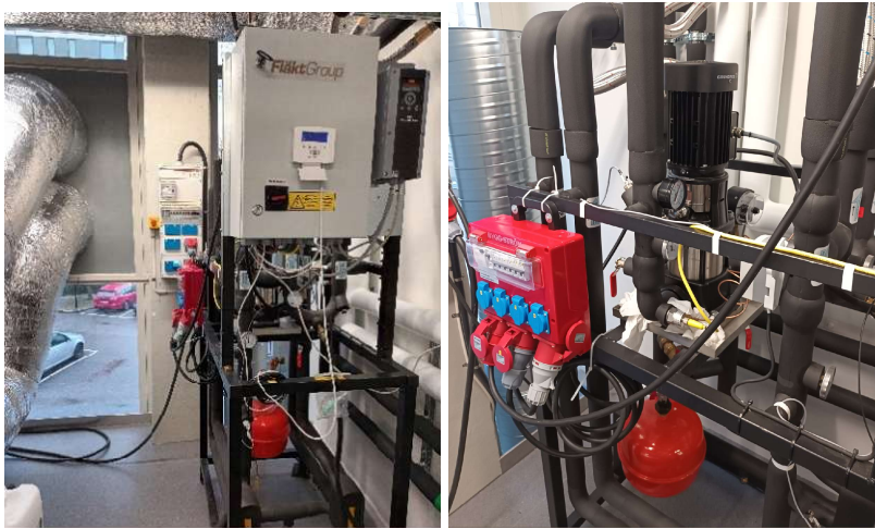
Figure 10: Pumping system of the RAHRU, photos taken in the laboratory.
