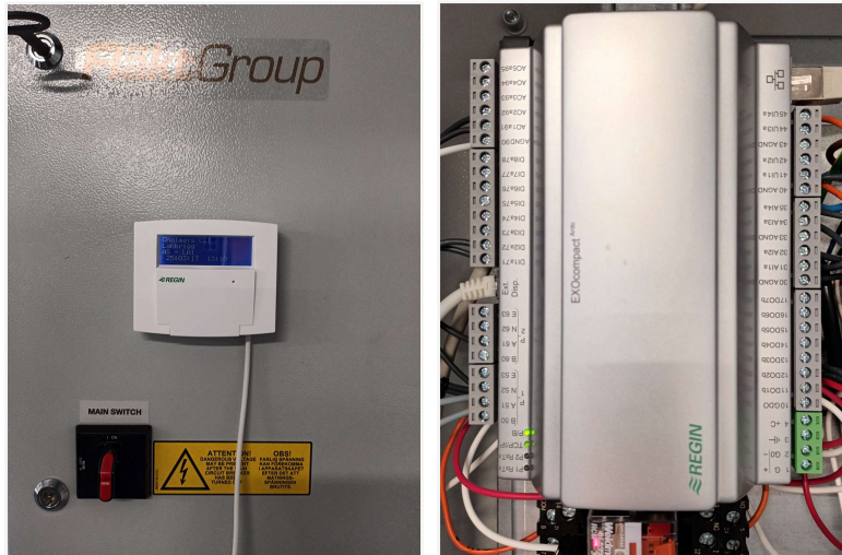
Figure 13: Field photos of the controller and its display unit.
