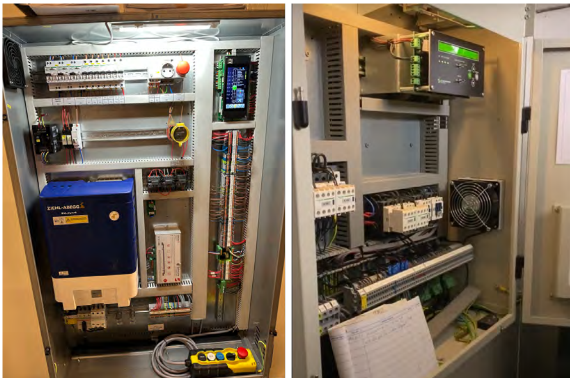
Figure 3.2: Control cabinets. Left: Photograph from lift fair. Right: Photograph from observation.
